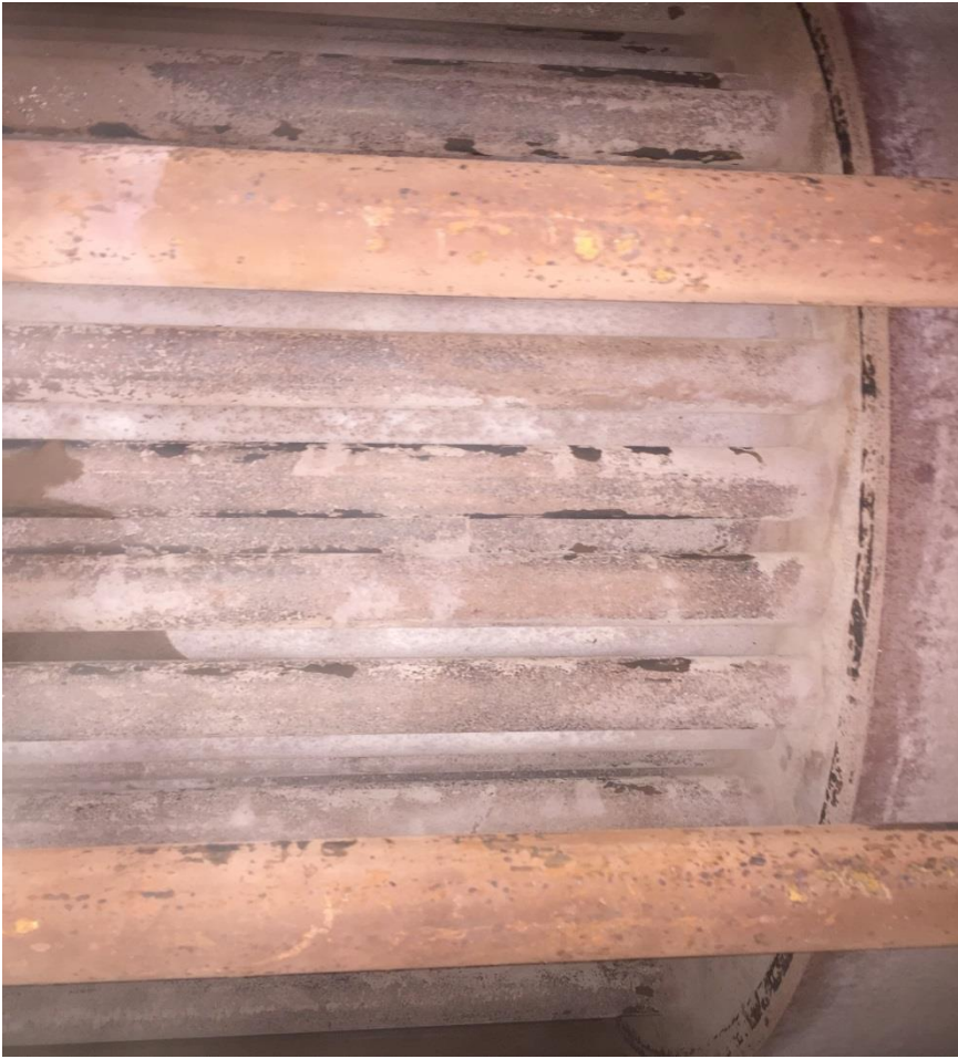
Boiler 2. Second and some third pass tubes and rear smoke box from top manway. June 2017
