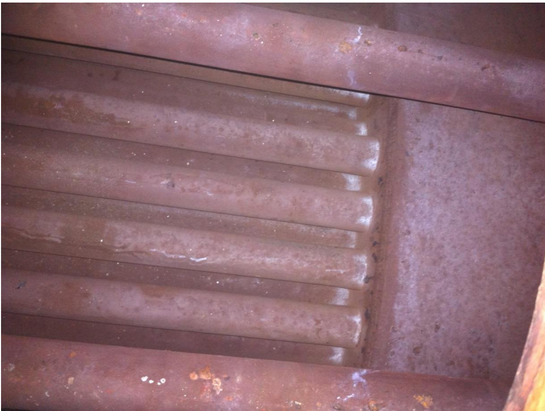
Boiler 2. Second pass and some third pass tubes and rear smoke box from top manway. June 2012
