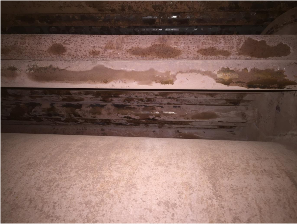
Boiler 2 Furnace, second and third pass tubes looking up through rear side inspection hole. June 2017
