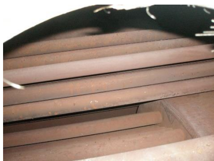
Boiler 2 Second and third pass tubes and rear smoke box from top manway. June 2013
