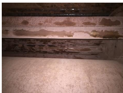
Boiler 2 Furnace, second and third pass tubes looking up through rear side inspection hole. June 2017
