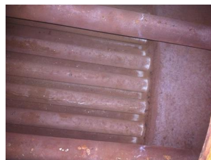
Boiler 2. Second pass and some third pass tubes and rear smoke box from top manway. June 2012
