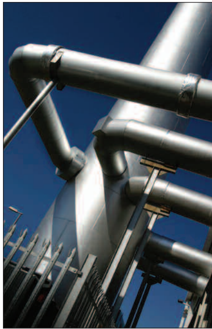
The flue serving the 1.4 MWe CHP energy centre at University Hospital Hartlepool.
