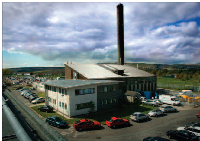
At the Prince Charles Hospital, Merthyr Tydfil, heating, hot water, and electricity, are provided by a 500 kWe CHP-based energy centre.
