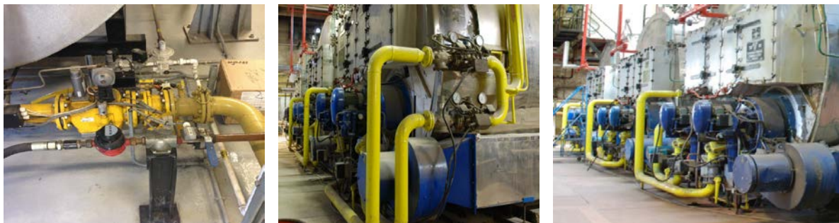
Above: Natural gas to boiler installations
