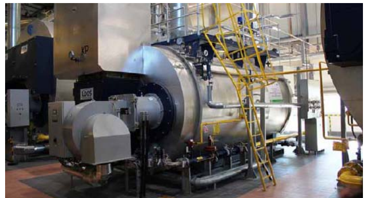
Boiler 2 1 x marathon® MC 10001.1 ARZsuper Combustion capacity 8 MW with Loos steam boiler UL-SX 10000x 10
