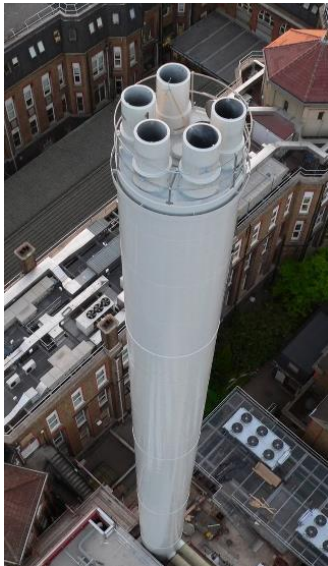
No matter how big or small your boiler plant - P roper P lanning and P reparation P revents P oor P erformance
