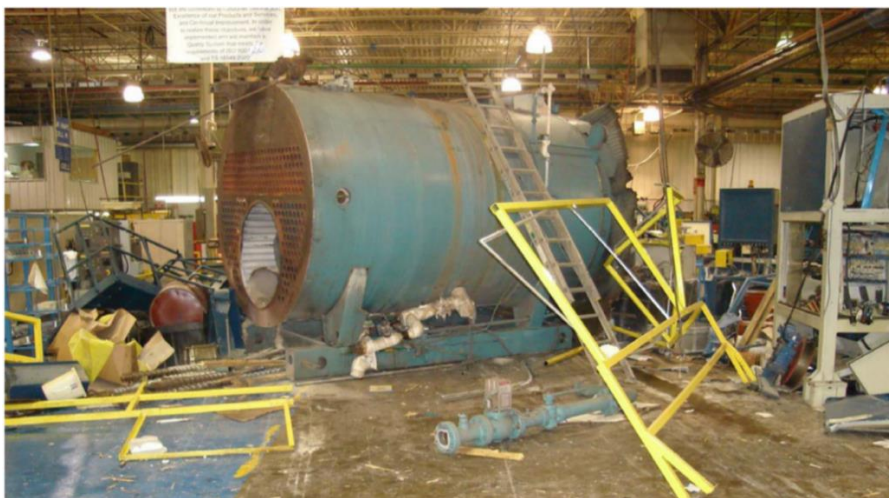
One possible outcome if maintenance isolations are not properly managed.
