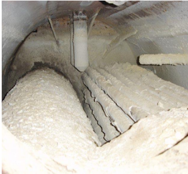
Above: Scale formation inside a boiler
