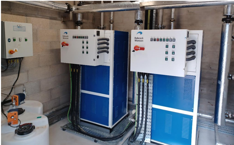
A pair of Babcock VAP-EL units installed within a group of 4 for a total installed power of 720 kW.
